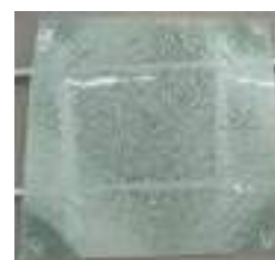
Figure 2: Fractured Façade Panel
